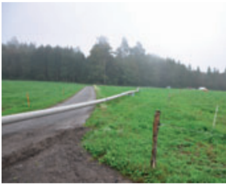
The pipeline had to be installed in rough terrain. Using a trenchless technique, about half of the 660 m long pipe string was laid under a forest, and the remainder under farmland.
