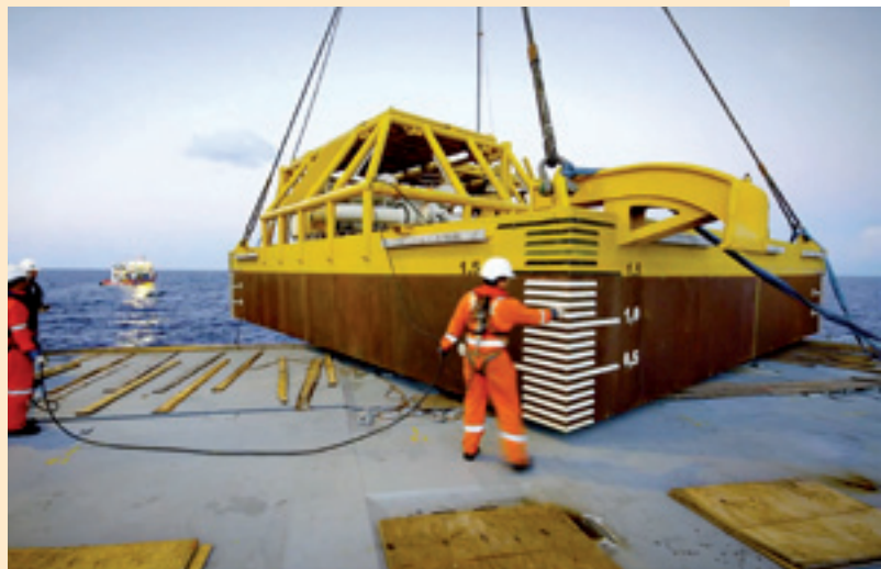
Top: The buoy a couple of hours before installation Bottom: Underwater installation of the pipeline end manifold (PLEM)
