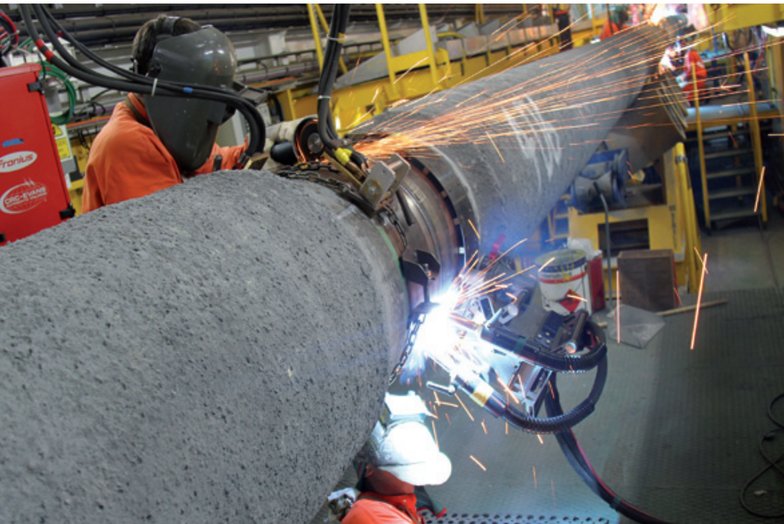
Micoperi welded the pipes into strings aboard a pipe-laying barge and laid the pipeline at depths of 50 to 80 m on the seafloor off the coast of Israel.
