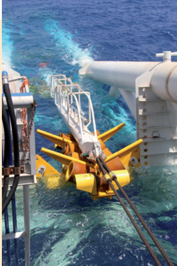
Laying the end of the 8 km offshore pipeline between the buoy and the national transmission system
