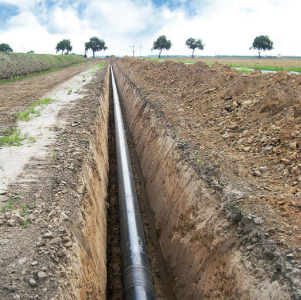
Project: Oxygen pipeline
