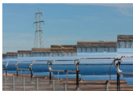
Parabolic trough power plants are among the most efficient and cost-effective concepts in solar energy power stations.
