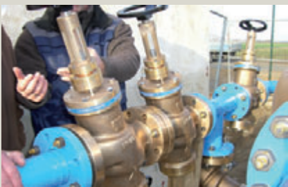
Top: View of Salzgitter Flachstahl GmbH Centre: The quality of the weld assumed special importance given that the pipeline is operated at a pressure of 30 bar. Bottom: Special valves control the operation of the oxygen pipeline.
