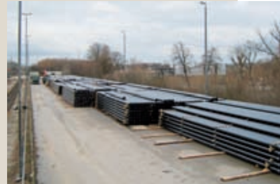
One of the large storage areas to which the pipes were delivered by rail. From here special trucks distributed the pipes along the route.
