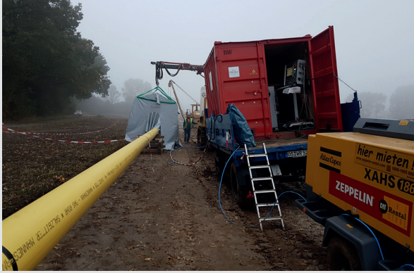
Figure 9: Construction equipment struggling with the mud
